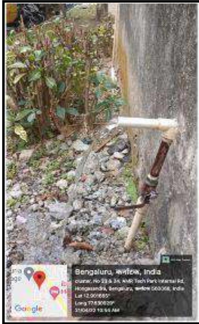
Figure 4-28: STP treated water tap for garden use
