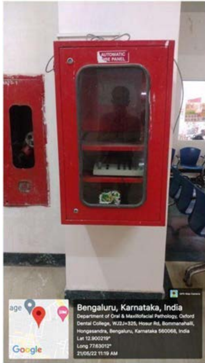
Figure 3-2: Fire alarm installed at ground floor- South wing
