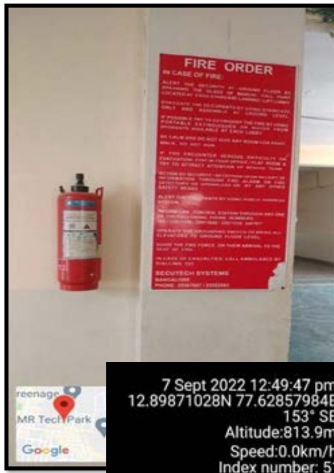
Figure 3-1: Fire order displayed at college premises
